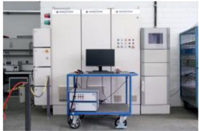
Figure 5: Control cabinets of the DC linearity test bench in the background, in front trolley with DPG10-4000B/F and PC
